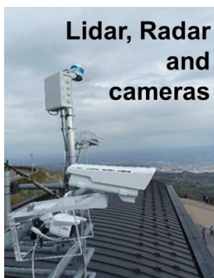
Figure 14 LiDAR RADAR and camera installation
